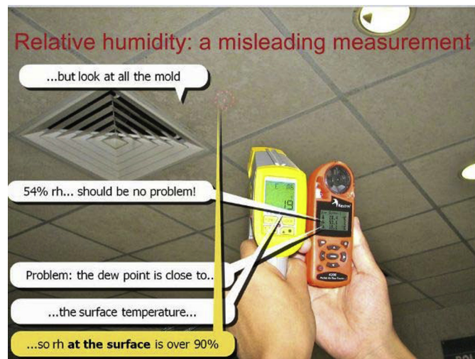
Figure 9. Temperature and humidity are not uniformly distributed throughout a house. The ceiling near the air conditioning supply vent has been chilled by the cold air to a temperature low enough to condense moisture and support dust mite and mold growth. Other locations inside a typical house may have similar micro-environments with excess or accumulated moisture.
